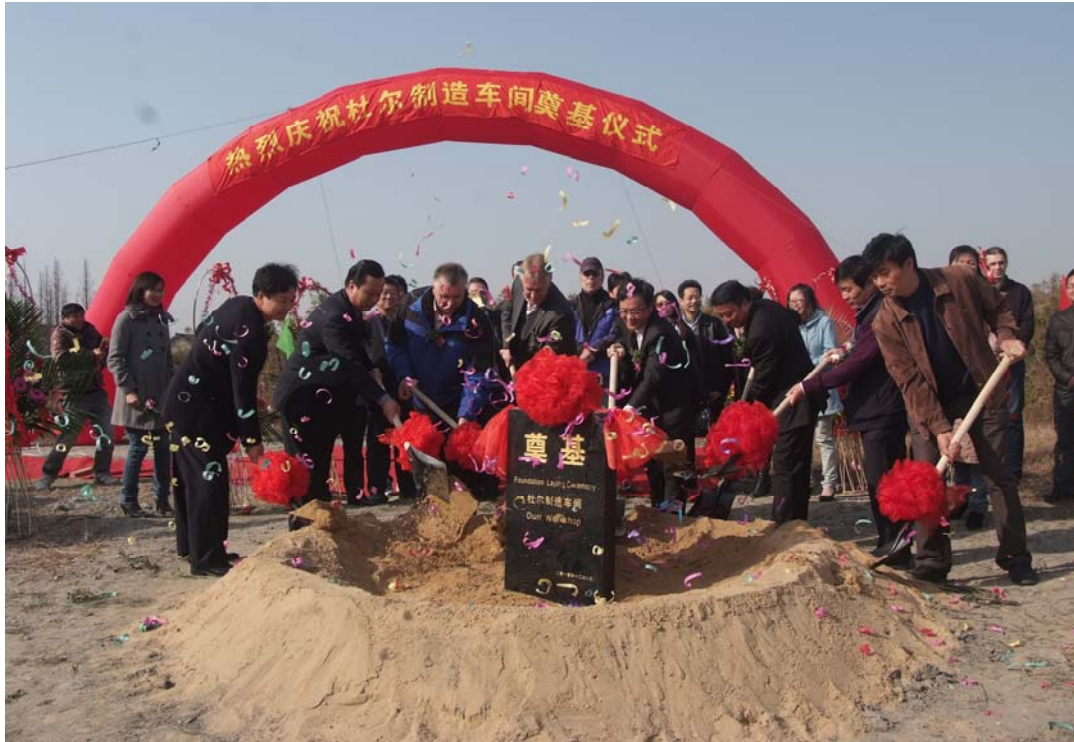
Honored guests starting foundation laying Left four Mr. Reiner Schmid, right four Mr. Jiang Ming, right three Mr. Yu Jianming
