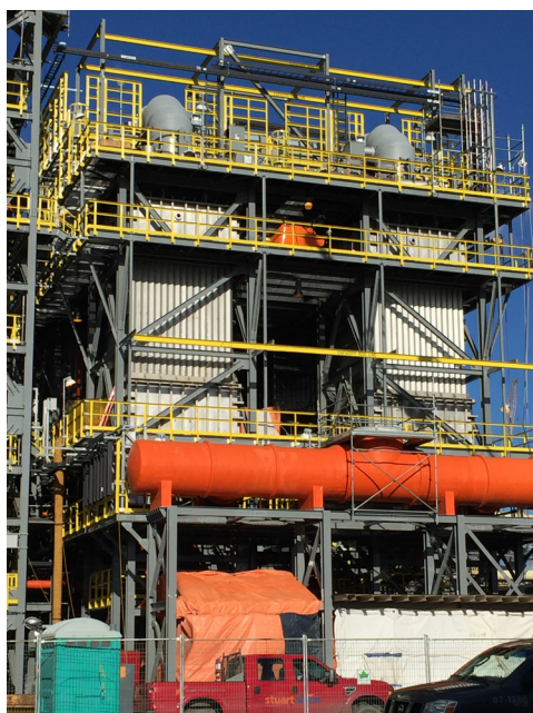
Installation of primary and secondary acid mist WESP trains for acid plant gas cleaning
