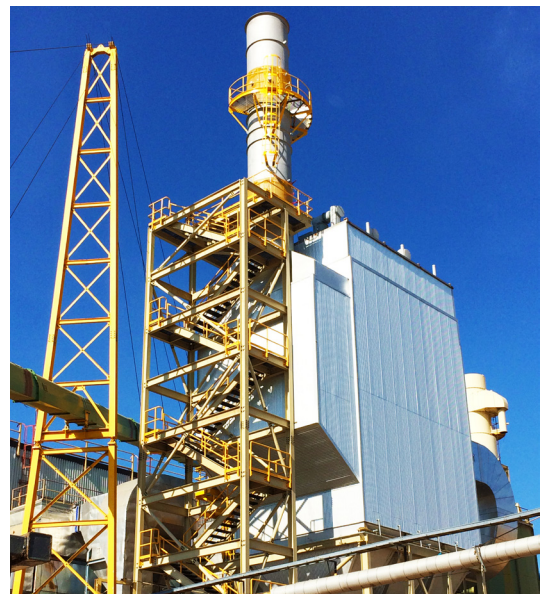
Proven process knowledge thanks to multiple installations
