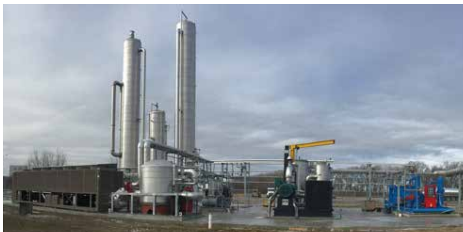
Installed 1,500 SCFM system with post-compression system.
