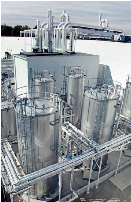
Solvent distillation column and tank farm
