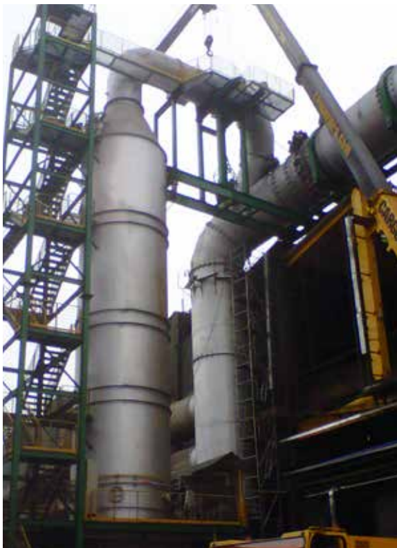
Evaporative gas cooling quench tower
