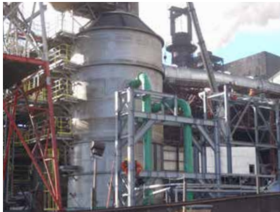
Wet scrubber for SO 2 control
